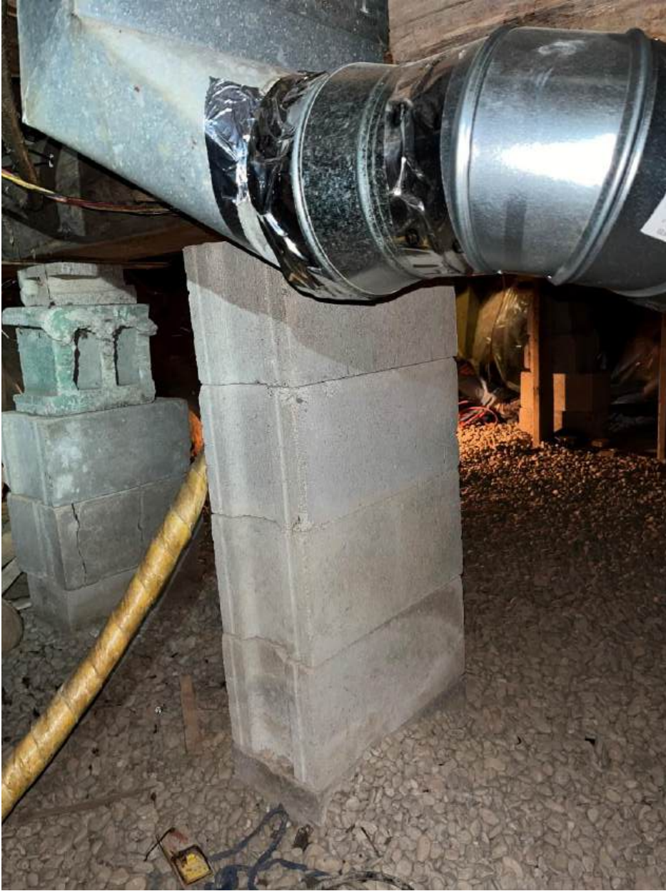
One stone pier – which appears precarious – will require work to stabilize.
