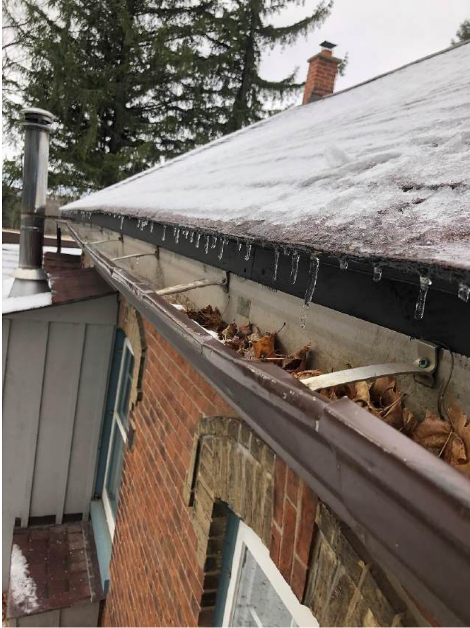
A cap is missing at the front end of the left eaves trough.
