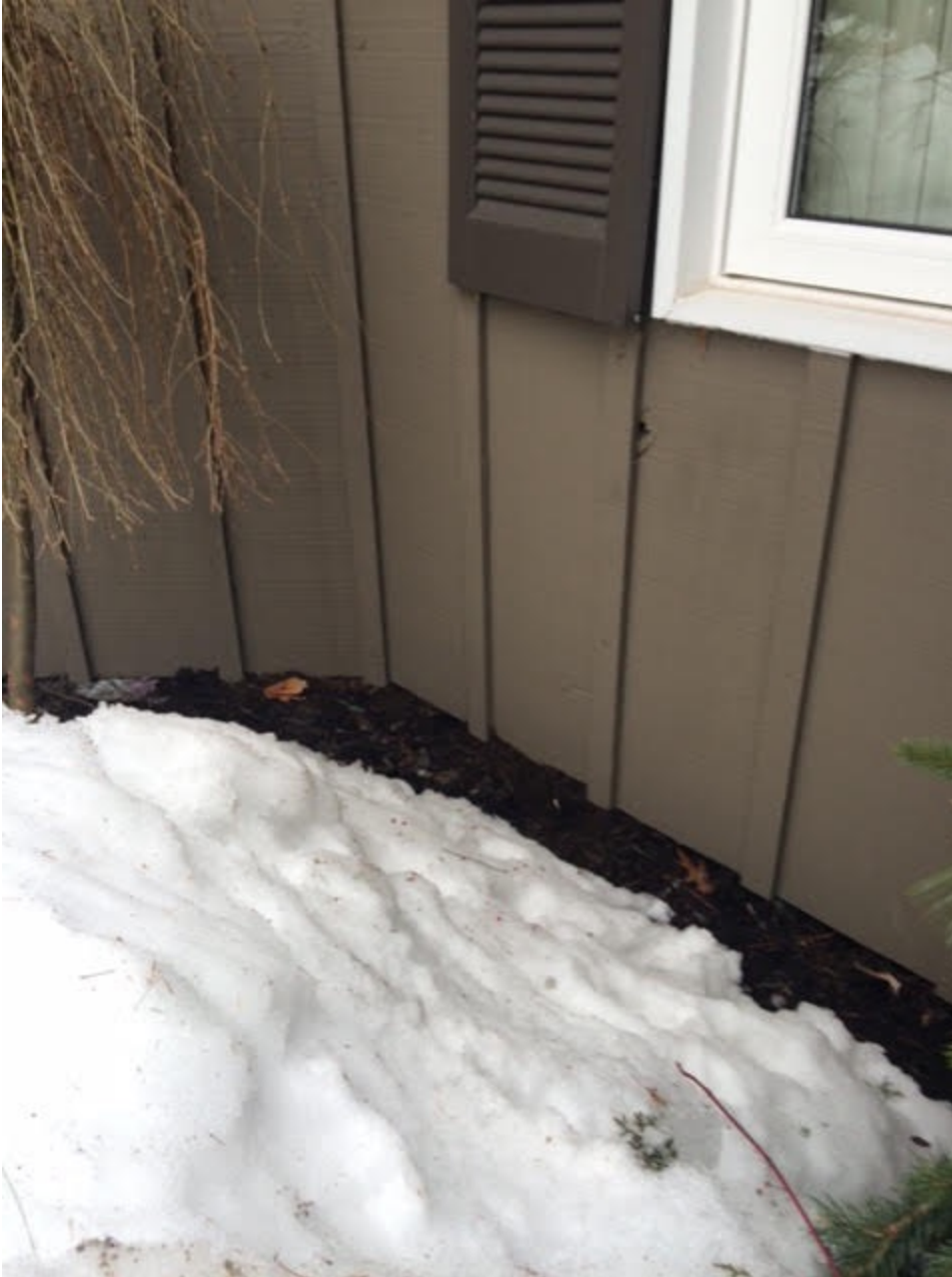
Settlement/stress cracks are observable at the left/front garage foundation wall, near the middle of the rear foundation wall, near the middle of the right foundation wall, and near the middle of the front foundation wall. (photos below)
